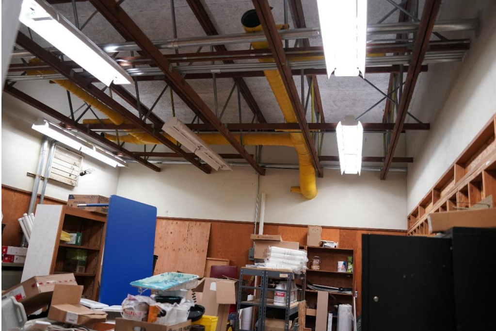
Figure 8 Wood shop duct collection ductwork.
