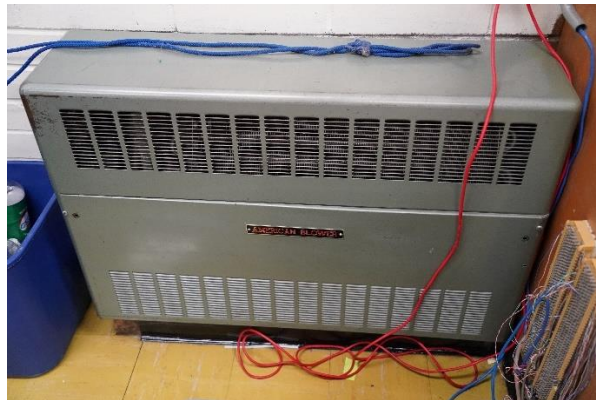
Figure 9 Office heating equipment
