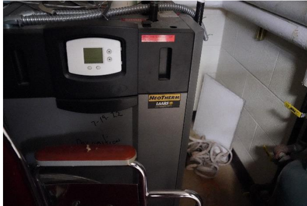
Figure 9 Decommissioned hot water boiler
