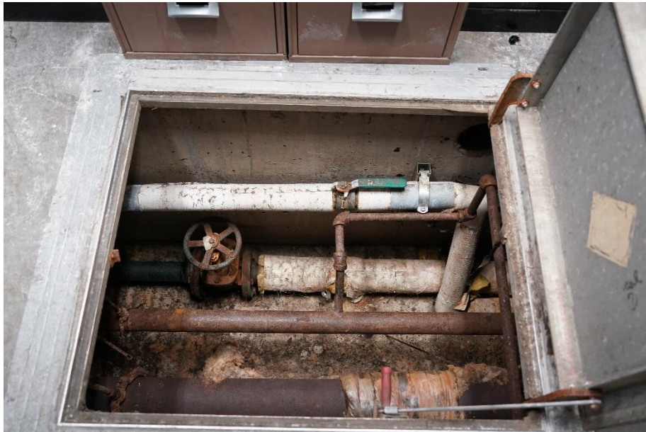
Figure 13 Steam and condensate piping tunnel/trench
