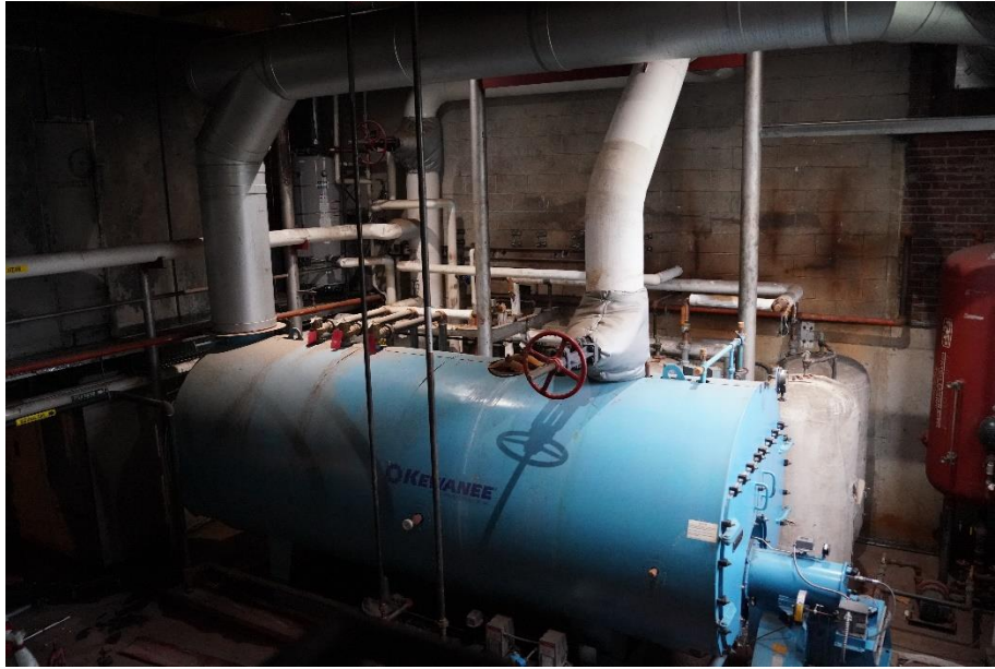
Figure 14 Failed steam boiler
