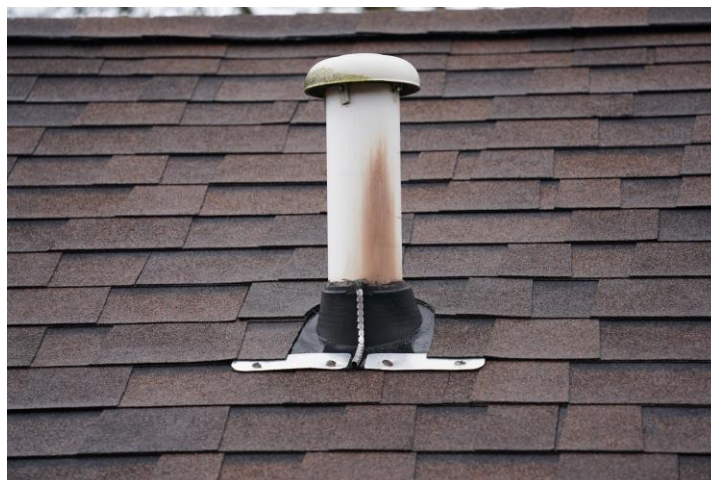
Figure 4 Gas vent pipe
