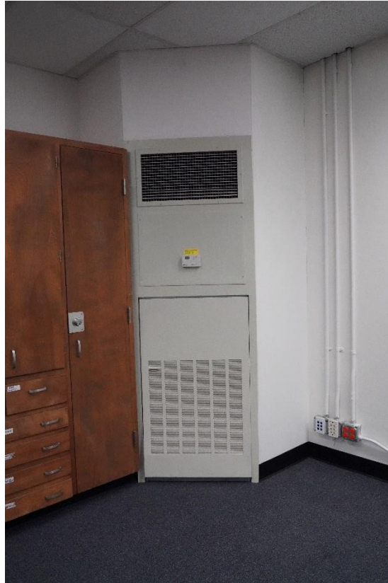
Figure 5 Abandoned in-place vertical fan coil unit
