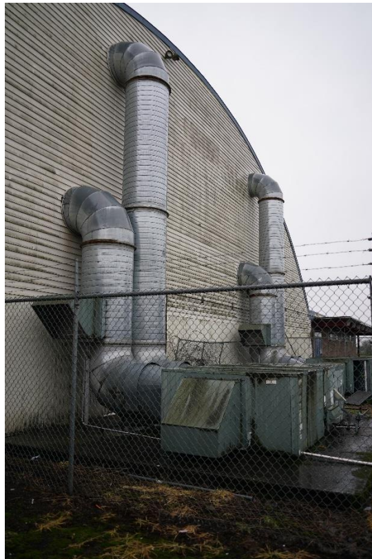
Figure 7 Gymnasium air handling units, AC-1 and AC-2
