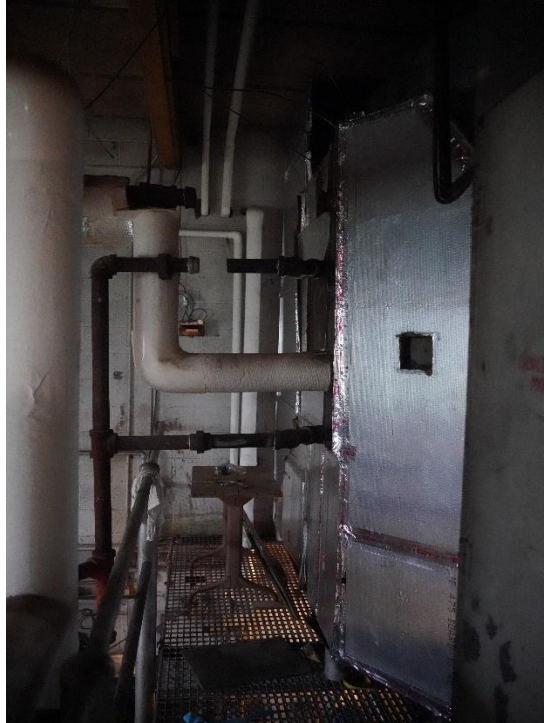
Figure 3 Original air handling unit, abandoned in place
