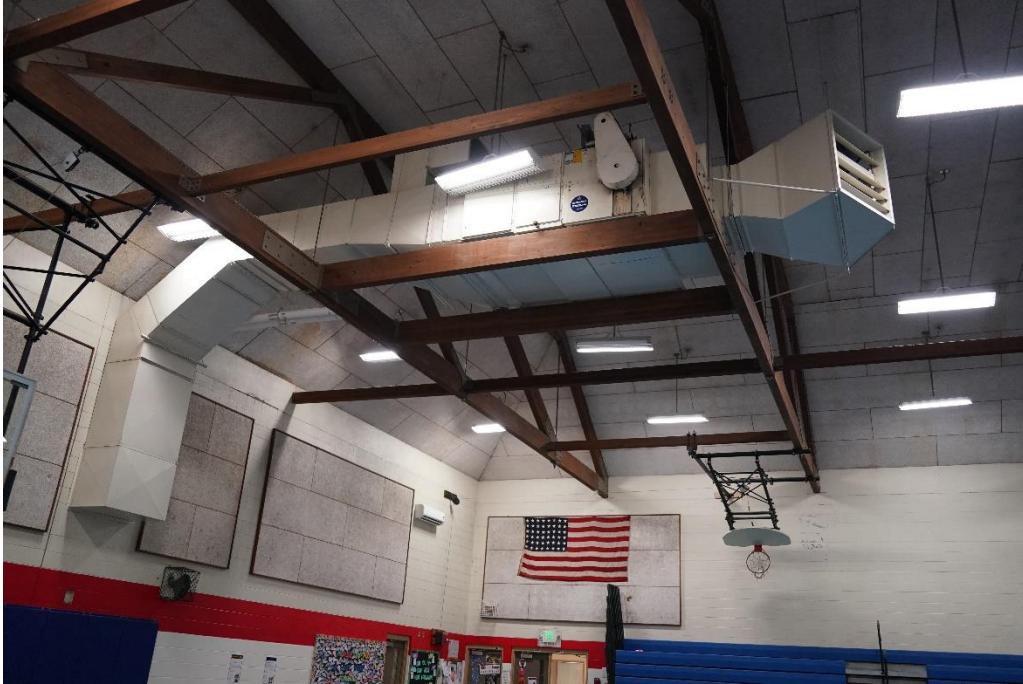
Figure 6 Gymnasium heating and ventilating unit
