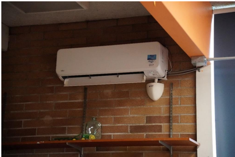
Figure 4 New classroom mini-split unit
