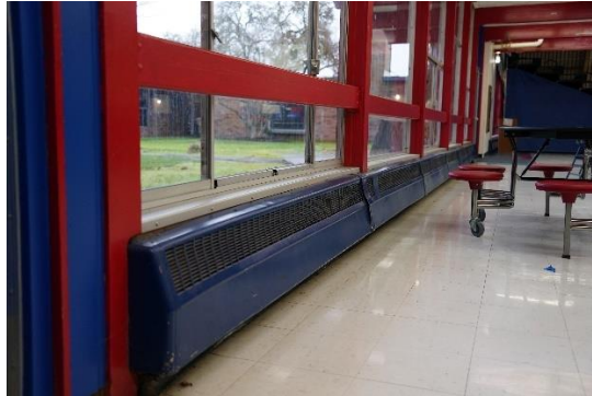
Figure 10 Lobby and commons heating equipment
